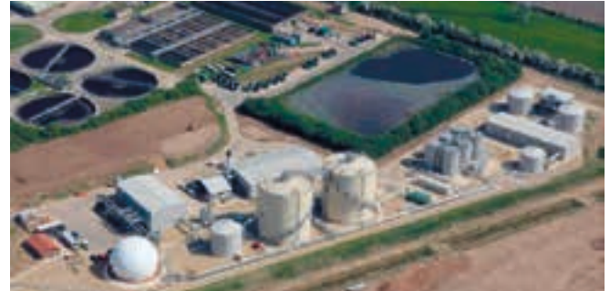
King’s Lynn Biosolids Treatment Centre (foreground) uses biogas CHP to generate sufficient power for the entire wastewater treatment plant.
