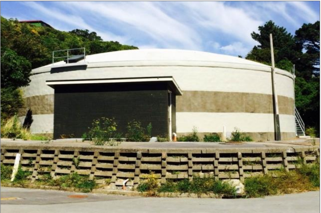
Photograph 2: Recent seismic upgrade works at Johnsonville reservoir (2.3ML). Works included wrapping and roof strengthening
