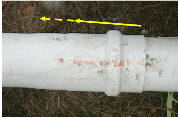
Figure X – Compressed ductile joint movement in PVC-u water main, Christchurch
