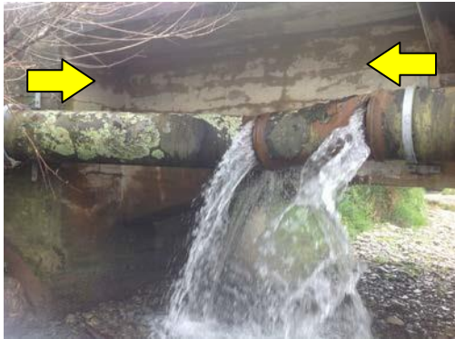
Figure V - Compression distortion and separation of RRJ joints in CLS watermain, axially aligned with the Eketahuna epicenter, 2014
