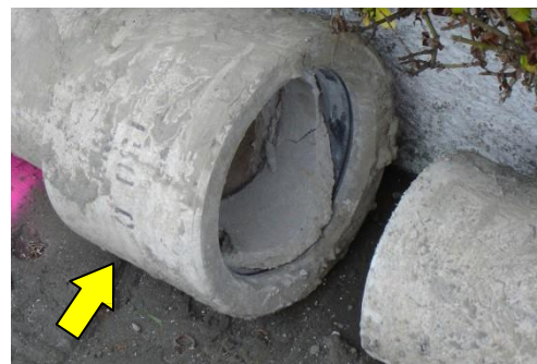
Figure VIII – Shear effects in AC pipe joint, Jollie Street, Kaiapoi, with tangential alignment to the Darfield epicenter, 2010
