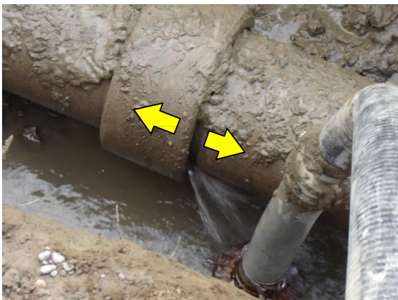
Figure III - Tension effects in AC pipe joint, Sewell Street Kaiapoi, axially aligned with the Darfield epicenter, 2010
