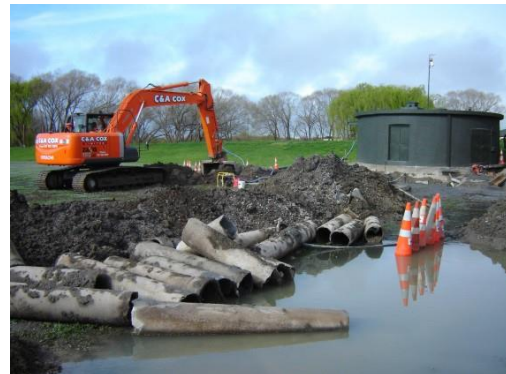
Figure VI – Compression fractures of pipe ends and joints in AC sewer rising main, Charles St, Kaiapoi, axially aligned with the Darfield epicentre, 2010 (Replaced with Biaxially Orientated PVC (PVC-O))
