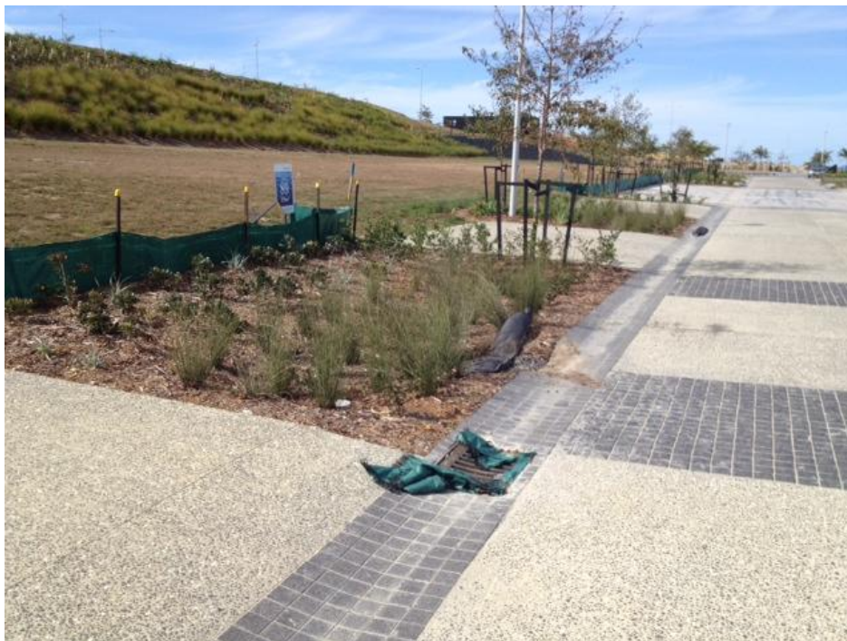
Photograph 3: Rain Garden Protection Features
