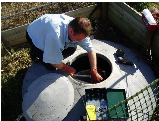
Servicing an advanced wastewater treatment unit
