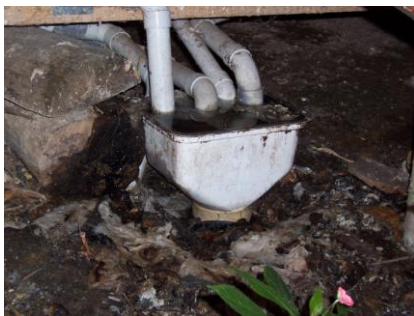
Backup to gully trap from clogged tank
