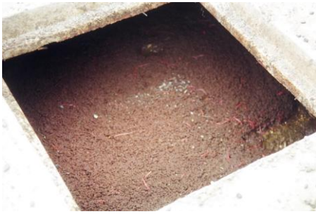
Healthy worm activity in septic tank scum layer
